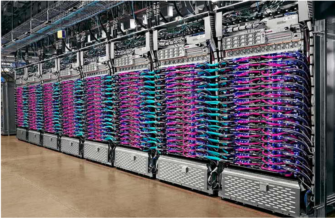
Figure 5: An eight-rack pod of Google's liquid-cooled TPU version 3 servers for artificial intelligence workloads. (Image: Google).
