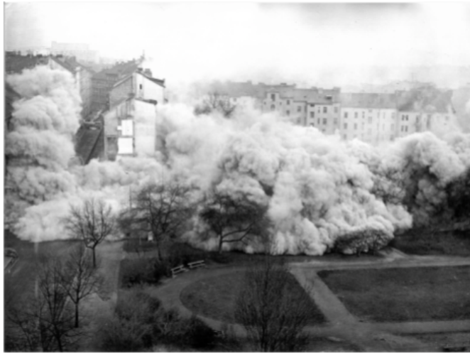
Image 7: Detonation of building complex in Žižkov, facing Vltkov Hill. By Jaroslav Kocourek.
